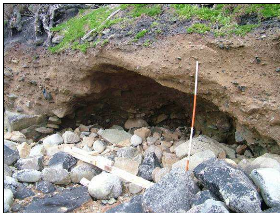
Fig 4.2 A cave 'large enough to hold a mini car' caused by sea wave erosion. Located to the west of King Charles' Battery (photo: EH)
