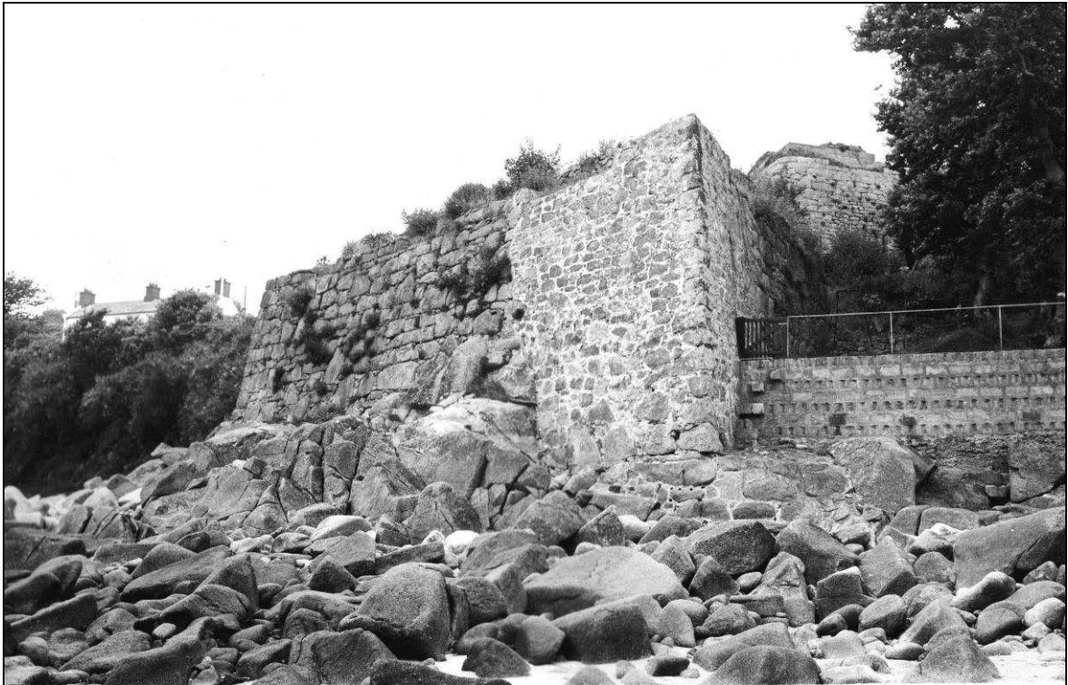
Fig 4.4 Lower Benham Battery (site 5) in 1972 showing an undated rebuild of the north-west 'right' part of the battery wall and also apparently a rebuild or repair of the north-east corner (photo: EH)
