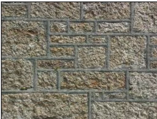
Granite ashlar with strap pointing on the former Bible Christian chapel, Church Street, 1899.
