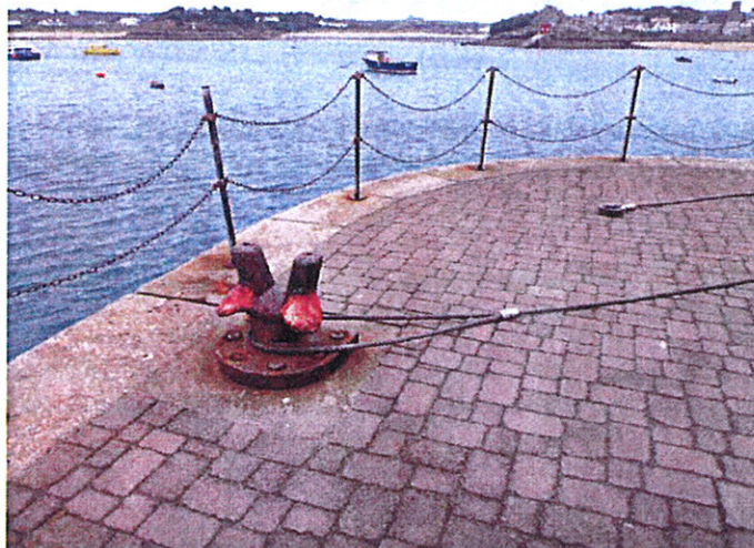
Photo showing End Bollard
