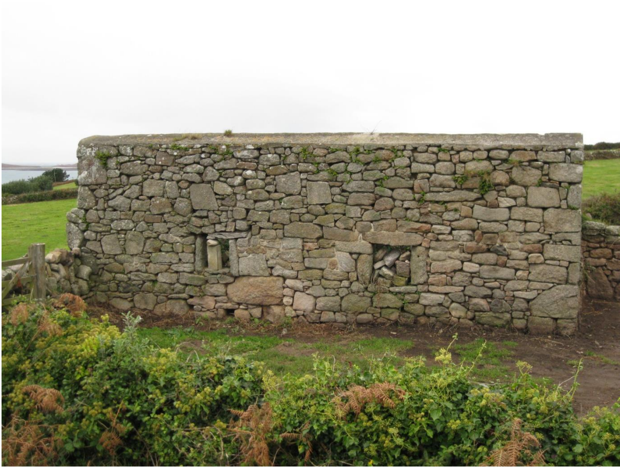
South elevation with rotted external timber lintel.
