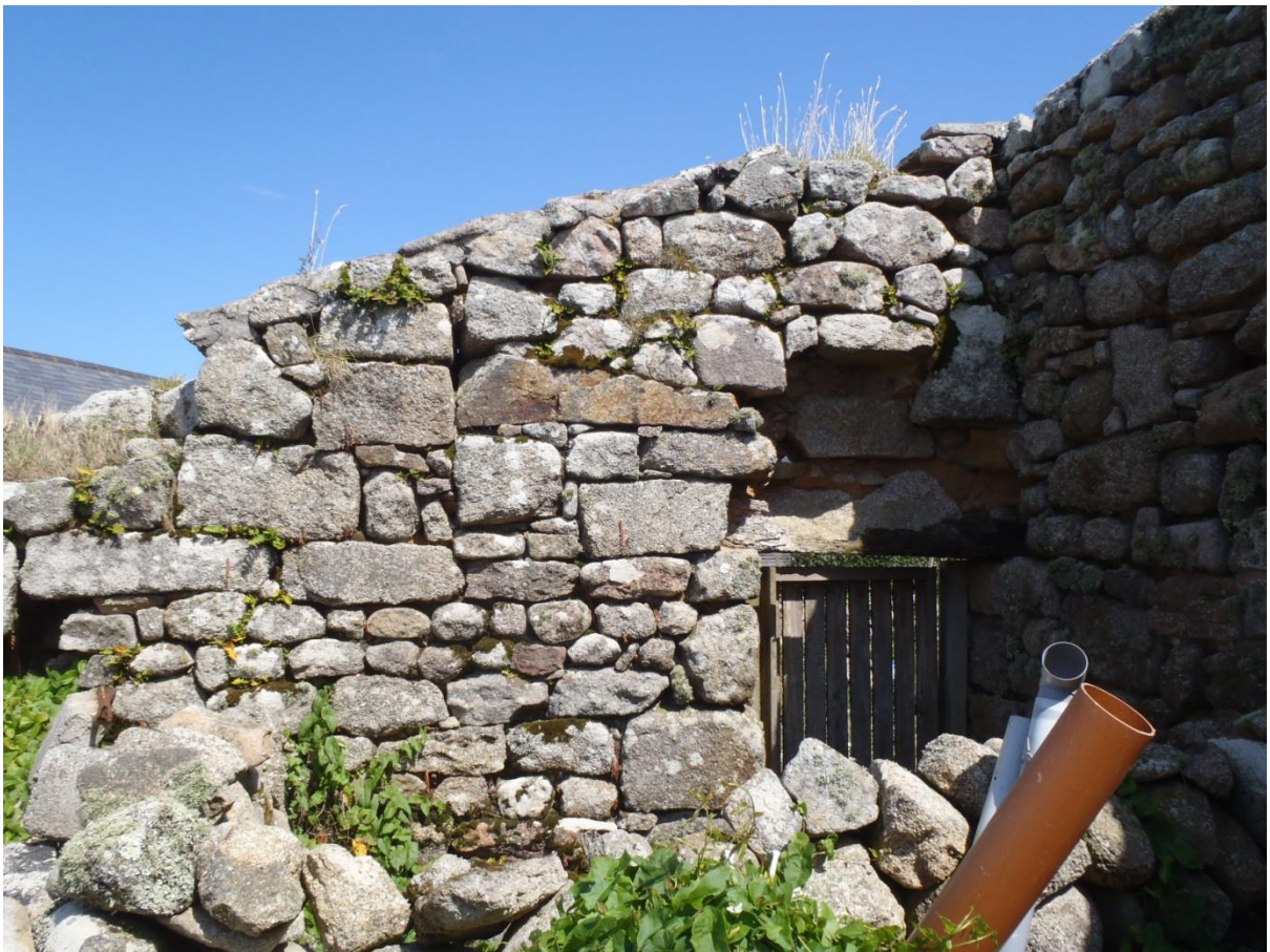
Internal doorway lintel rotted away
