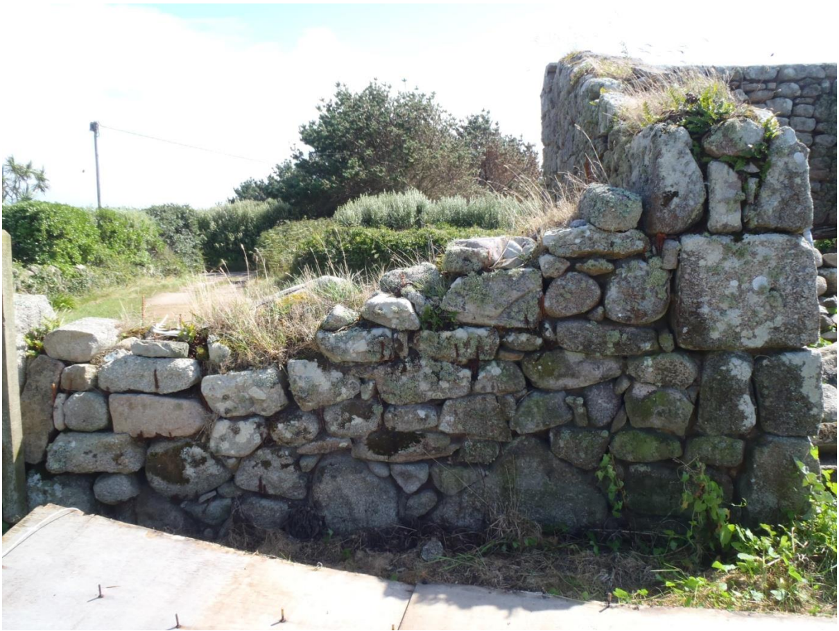
An example of how the stone work is not easy to read
