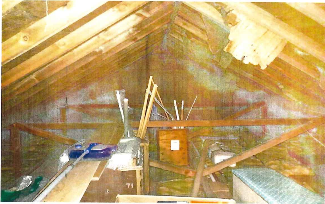
Photo 7. Loft space showing collar beams and ridge board joints and tears in the lining.
