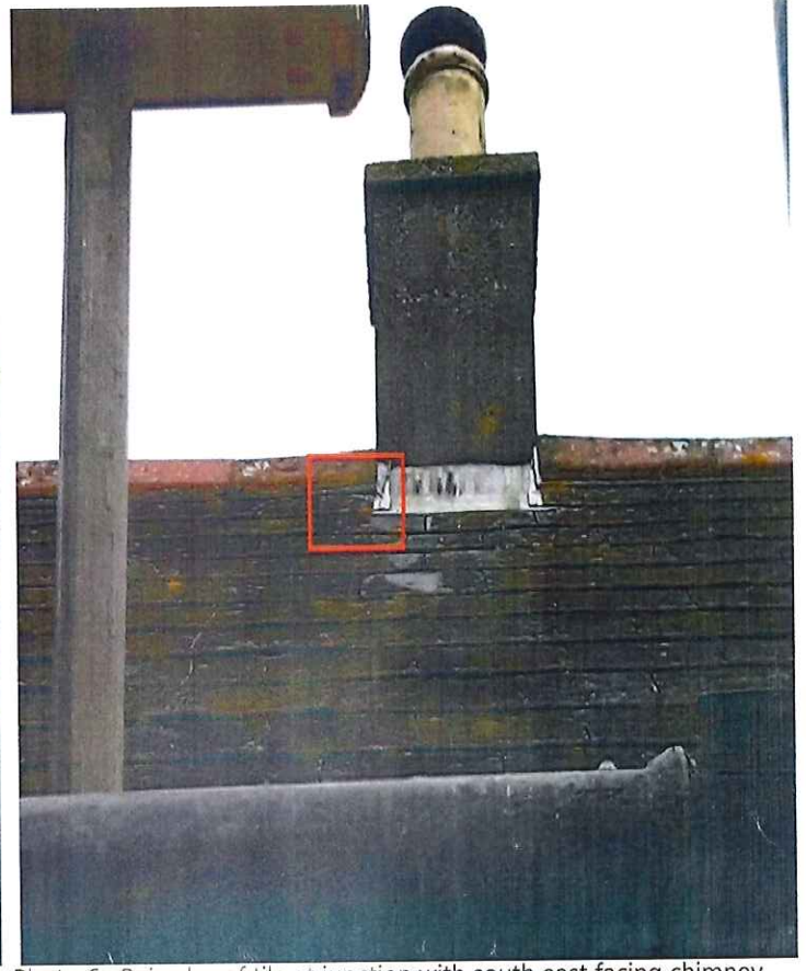
Photo 6. Raised roof tile at junction with south east facing chimney
