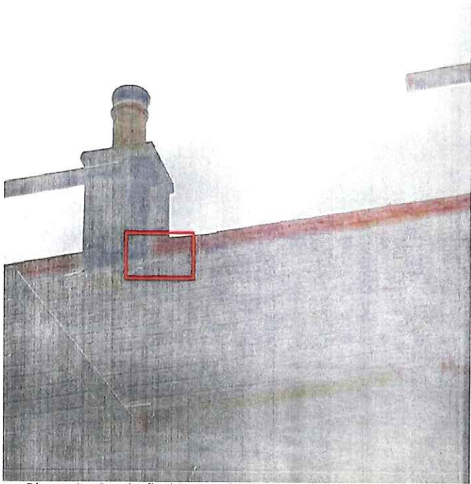
Photo 1. Gap in flashing and raised roof tile
