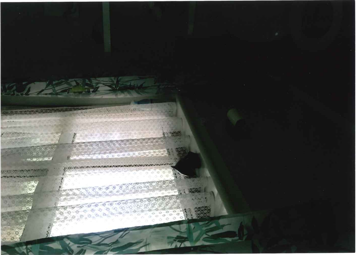
EXISTING WINDOW DOES NOT LIGHT ROOM DUE TO COVERED WALKWAY OUT SIDE - LIGHT NEEDS TO BE PUT ON (AS IN PHOTO ABOVE)
