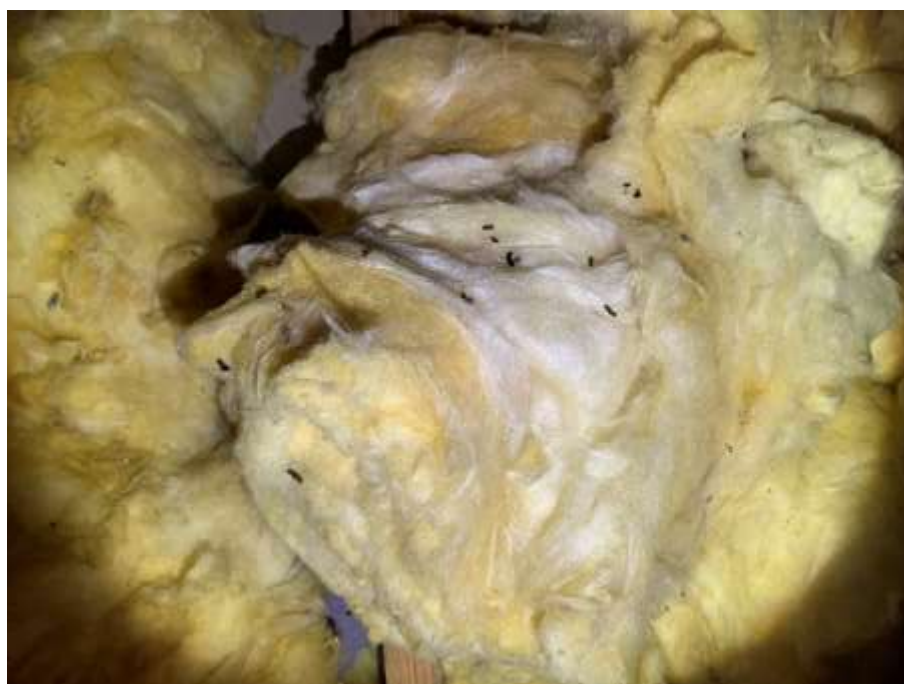
Figure 10: View of the bat droppings scattered throughout the roof void.
