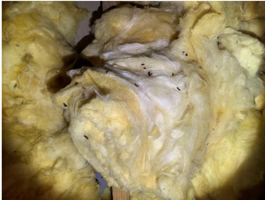
Figure 6: View of the bat droppings scattered throughout the roof void.
