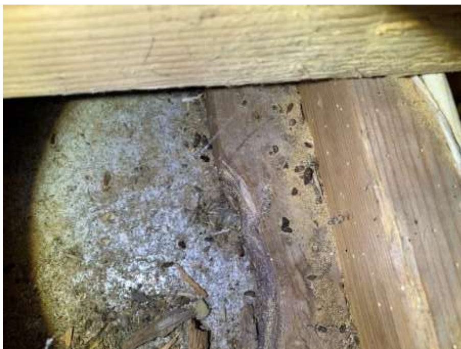
Figure 11: View of the cluster of bat droppings found beneath the internal chimney breast.
