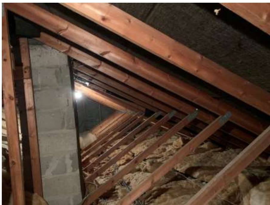
Figure 9: Interior view of the fink structure roof void; bitumen lined and rolled insulation between the joists within Racket Town.
