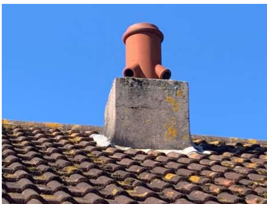
Figure 8: View of the concrete chimney and gaps beneath the lead flashing.
