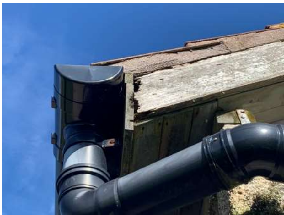
Figure 7: View of the rotten wooden fascia on the south-west corner of Racket Town.
