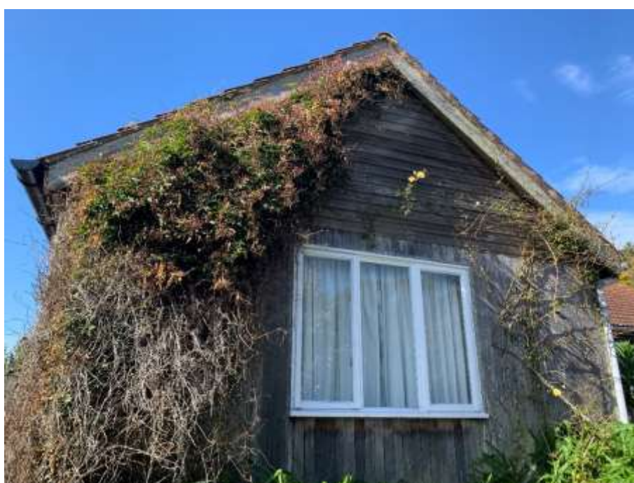
Figure 4: View of the eastern elevation of the projection of Racket Town, showing dense ivy.
