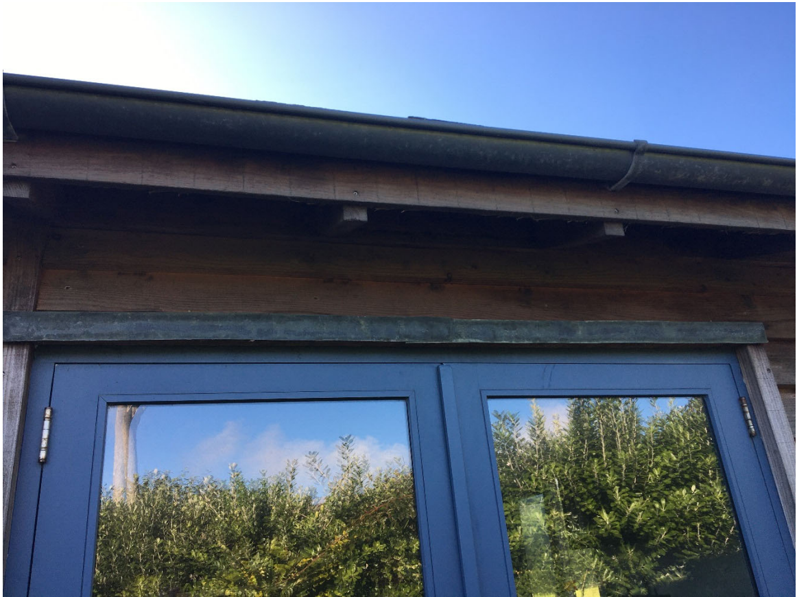
Roofline where the new Work Room will be connected to Island Fish
