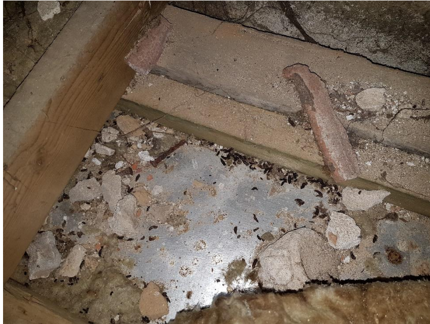
Figure 11: Accumulation of bat droppings at the northern gable end within roof void over the apartment.
