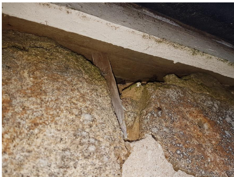
Figure 9: Gap on wall top behind fascia board on western elevation
