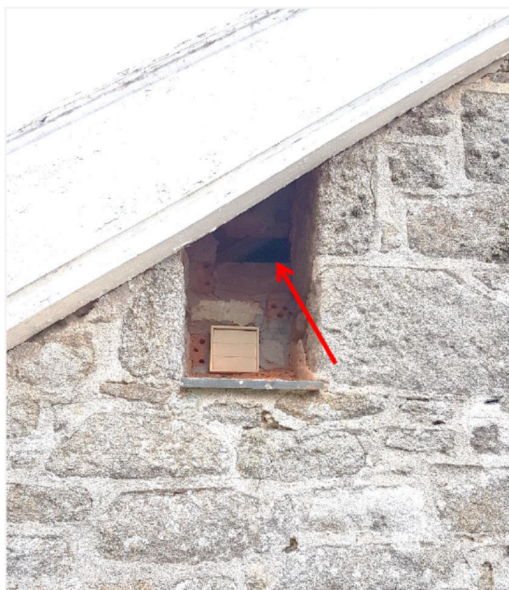
Figure 8: Gap under eaves on southern gable end
