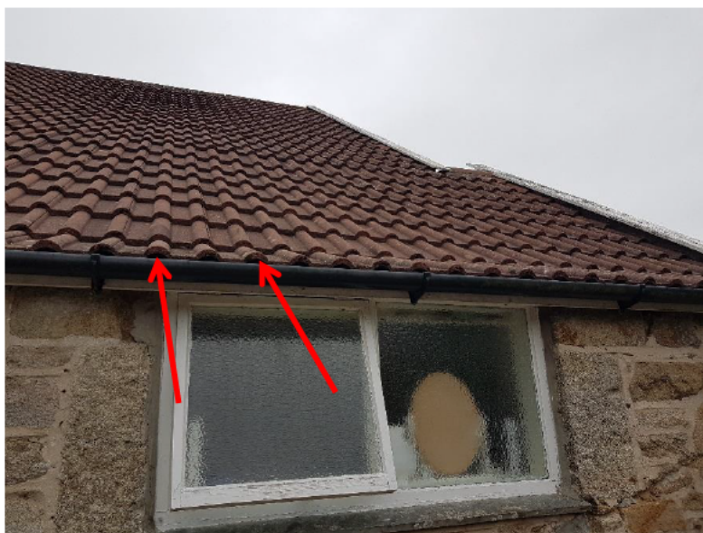
Figure 7: Gaps underneath the interlocking roof tiles on western elevation
