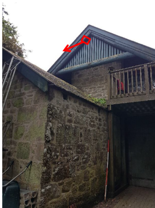
Figure 16: Location of a brown long-eared bat seen to emerge during the second emergence survey (red arrow) under wooden fascia near the apex on the northern elevation of Valhalla.
