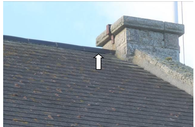
Photograph 4: Showing one of the minor gaps beneath the ridge tiles on the hall.
