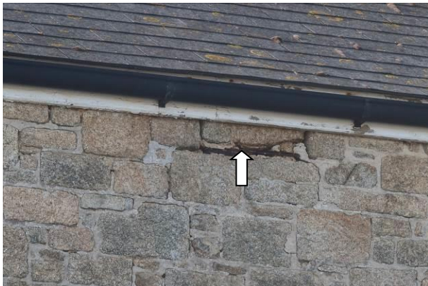
Photograph 3: Showing one of the cracks in the blockwork on the eastern aspect of the hall.
