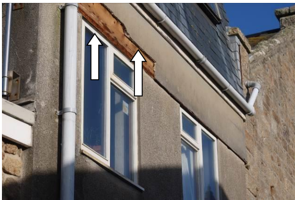
Photograph 9: Gaps behind the boarding on the southern aspect of the 1970's extension; similar features are present on the western aspect.
