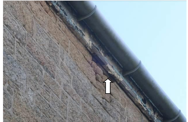
Photograph 2: An example of the gaps behind the fascia board on the western aspect of the hall as well as gaps in the pointing beneath.
