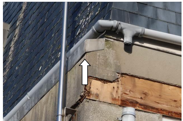
Photograph 10: Showing an example of lifted flashing between the slate tiles of the Mansard roof and the boarding beneath on the 1970's extension
