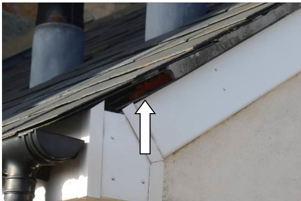
Photograph 5: Showing an example of the gaps allowing potential access beneath slate tiles in the plant room; similar features exist on the rear porch.
