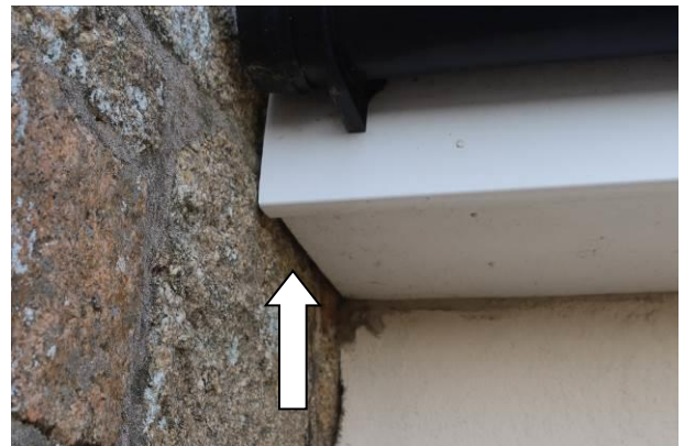
Photograph 6: Showing an example of the gaps allowing potential access beneath soffit box in the plant room; similar features exist on the rear porch.
