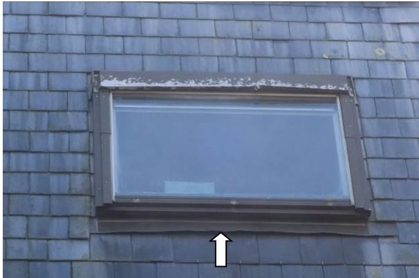
Photograph 1: Showing the lifted flashing around the window on the 1970's extension on the northern aspect.
