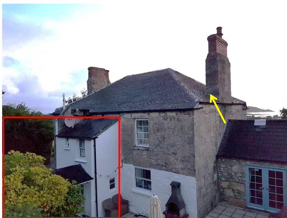
Figure 9: Re-entry location of a single common pipistrelle bat into a gap under lead flashing on the south western elevation of the south eastern chimney on 28 th August 2020 (yellow arrow). Red outline shows approximate extent of proposed works at Dolphin House (including outbuildings further to the west).
