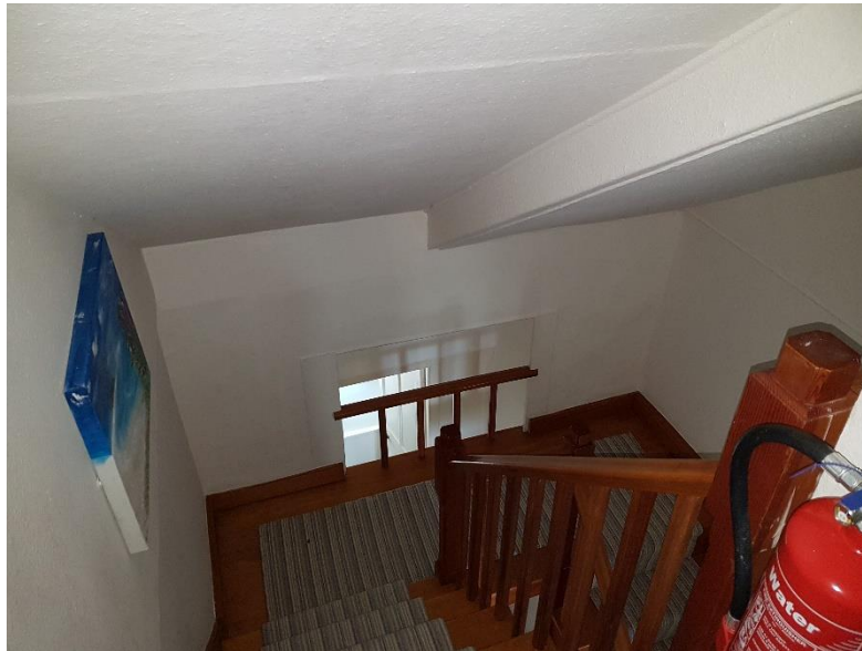
Figure 6: Interior of second floor stairwell within Dolphin House (viewed towards the south-west)
