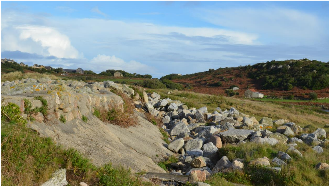
Figure 1-5: Dilapidated sea wall at Great Popplestone
