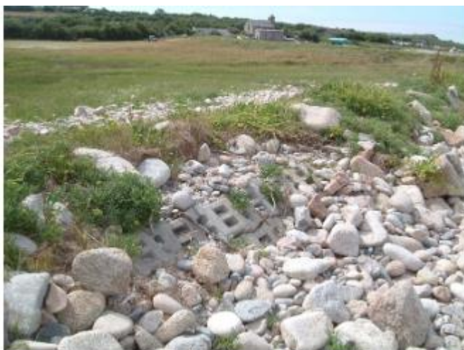
Figure 4-30: Backshore condition after winter storms (JLA 2014)
