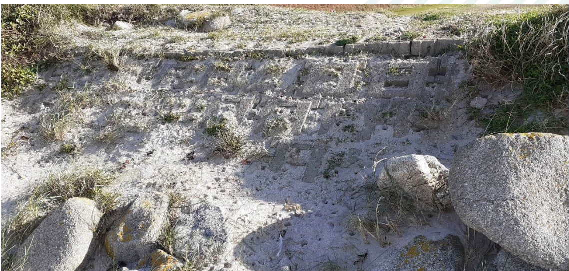
Photograph 21: Area of exposed concrete sea wall (MCO64519)
