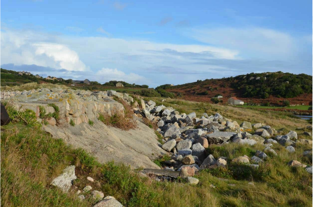
Photograph 15: displaced rock and soil revealing concrete face of Great Popplestone coastal defences
