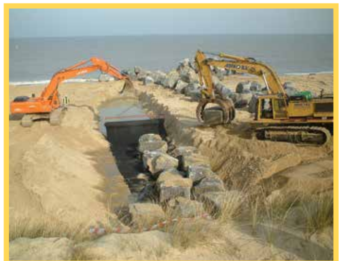
Rock armour Groyne installation to inhibit 'Long Shore Drift' and protect the coastline.
