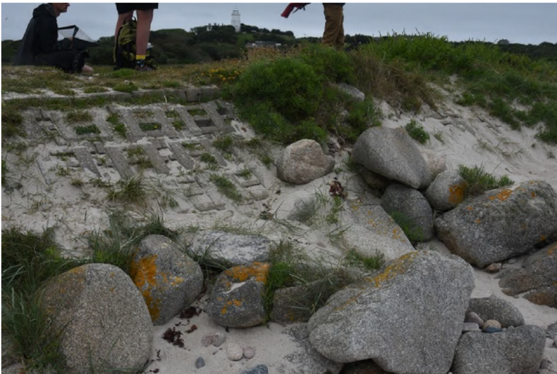
Photograph 2 – Armourflex concrete mattress fronted by large boulders
