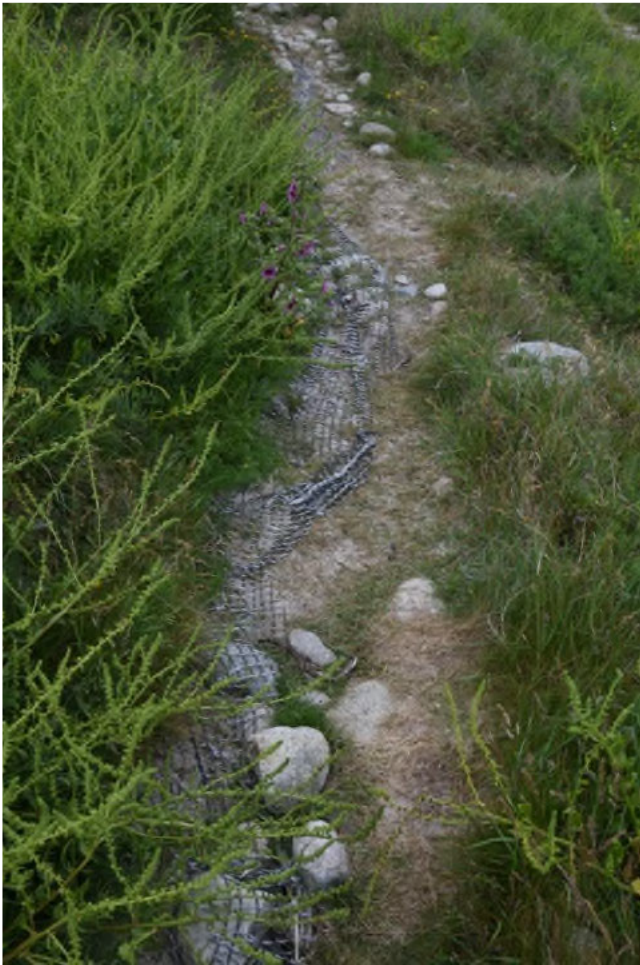
Photograph 6 – Exposed mesh on the ridge
