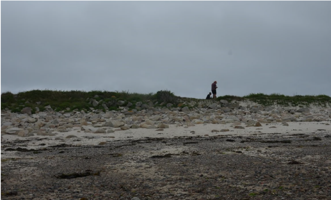
Photograph 1 – View of the ridge armoured with the Armourflex concrete mattress, fronted by boulders, at its toe, and a layer of cobbles and gravel over the beach
