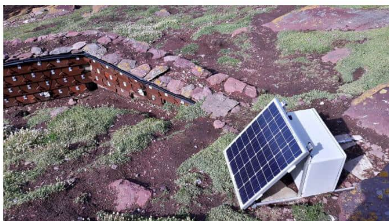
The solar control box. Chris Payne
