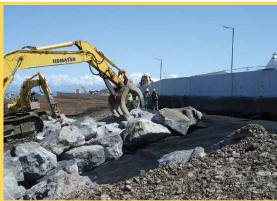
▲ Typical primary rock armour revetment installation directly on HPS geotextile. Location: Colwyn Bay.
