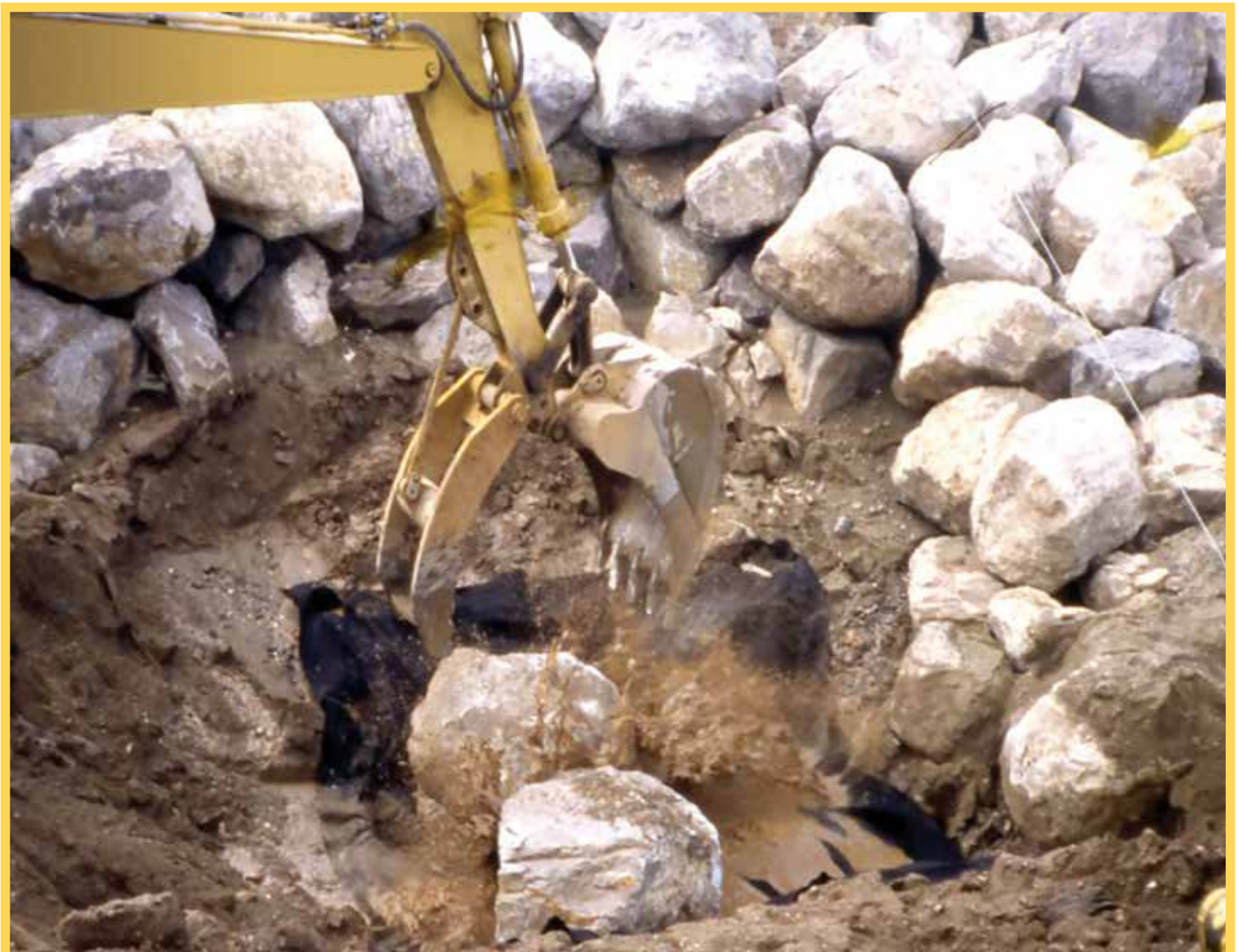
▲ Live Installation: 3t rock armour dropped from 2m height onto HPS14 overlying a sandy clay unconsolidated beach deposit.
