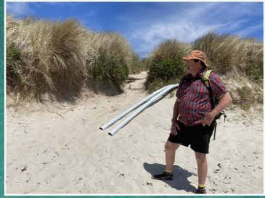
I SITE 26. Location of exposed cables dune erosion
