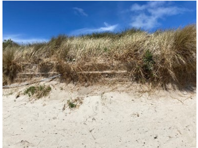
Figure 6.2: Exposed cabling at top of the beach
