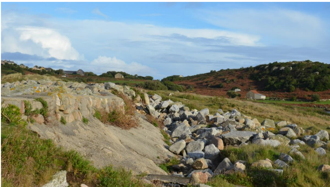
Figure 4: Run down sea wall at Great Popplestone.
