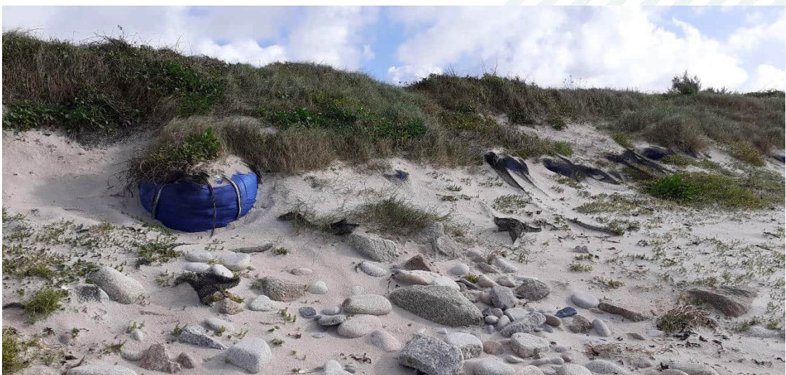
Photograph 24: Exposed geobags due to erosion of the bank
