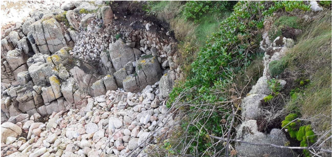
Photograph 18: Area of erosion at Porth Killier where the 'fan-shaped' rock armour is proposed
