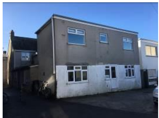
Photo 07 - Showing the northern and eastern facades of Building C. The flat-roof Building B can be seen on the left-hand side with Building A behind.
