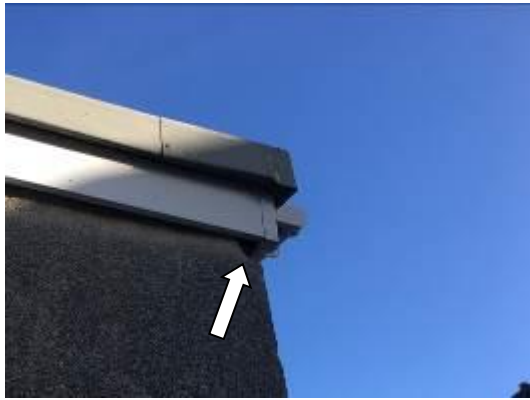
Photo 10 – Showing the fascia on the southern aspect of Building C with a gap visible on the south-eastern corner.
