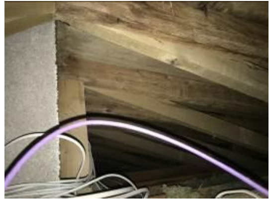
Photo 05 - Showing the view into the loft space of Building B as seen from the small hatch
