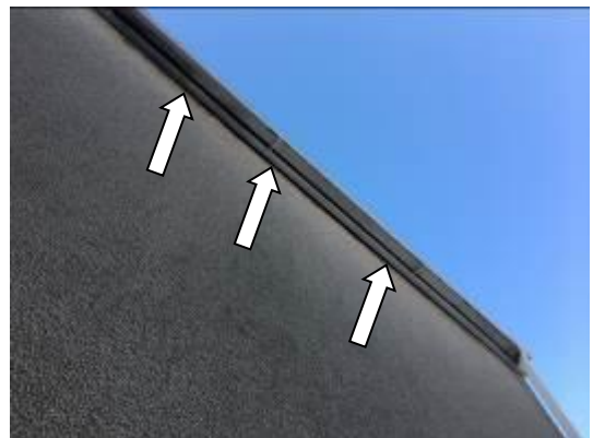
Photo 09 - Showing the fascia board at the top of the walls on Building C - gaps occur in places, predominantly on the eastern aspect.
