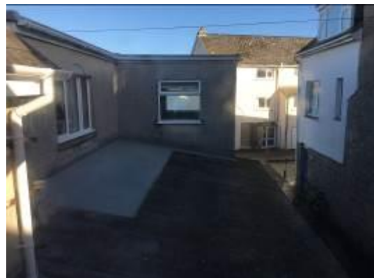
Photo 03 – Showing the gently-pitched fibreglass roof of Building B from an elevated viewpoint. Building C is present in the background and on the left-hand side.
