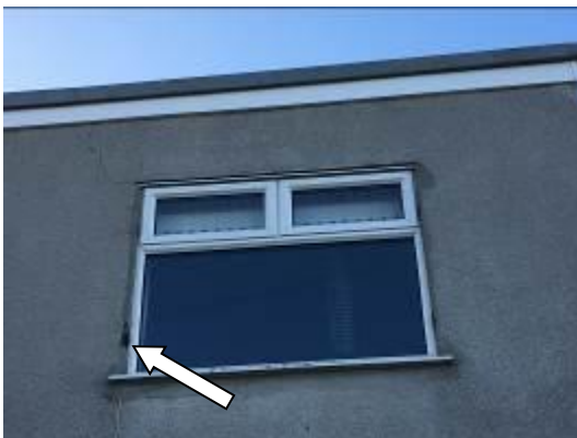
Photo 08 - Showing an example of the cracks/damage which occur occasionally in the render of Building C - these do not appear to offer roosting opportunities. Both the uPVC and wooden windows are largely well-fitted with no gaps noted.
