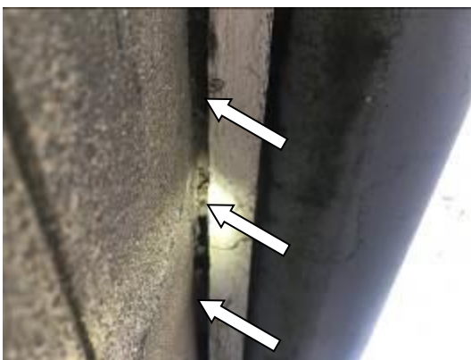
Photo 06 - Showing an example of the gap behind the fascia board on Building B which is likely to provide potential access for bats to the internal roof void.
