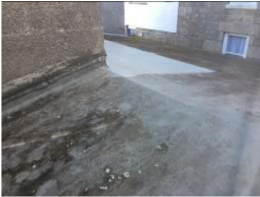
Photo 04 - Showing the typical well-sealed flashing where Building B connects with Buildings A and C at either side
