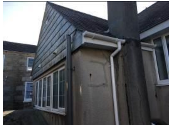
Photo 11 – Showing the northern aspect of Building A which directly faces Buildings B and C. The hanging tiles are tightly fitted and no gaps were noted on this aspect.
