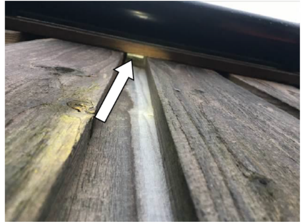
Photograph 2: Showing the gap behind the fascia board at the eaves – however this is open at the top with no apex cavity which would reduce its suitability for use by roosting bats.
