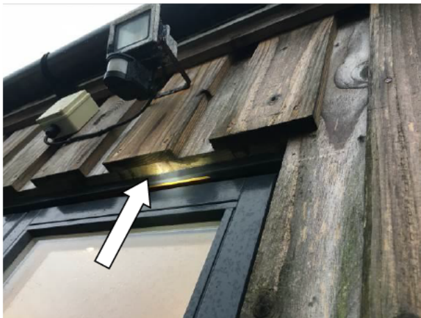
Photograph 3: Showing that the potential gaps in the hit & miss have been sealed above the window.
