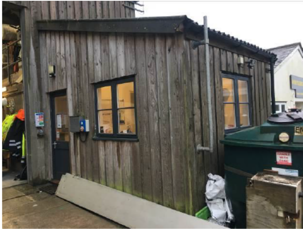
Photograph 1: Showing the office unit – the northern face would be removed to allow the building to be extended over the footprint of the existing oil tank (visible to the far right).
