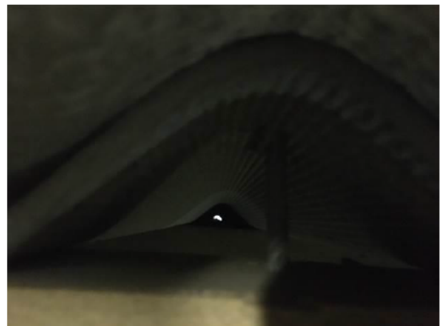
Photograph 6: Showing view along the corrugated roof sheet from the interior of the warehouse – the light is visible at the end in some instances only.
