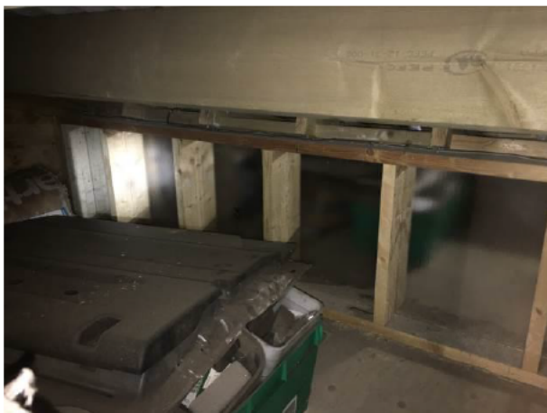
Photograph 5: Showing the accessible portion of the void as seen from the warehouse – the CLS internal structure and insulation boards are visible.
