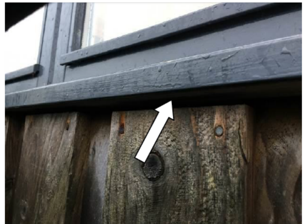
Photograph 4: Showing the very minor cavity below the sill of the aluminium window frame.
