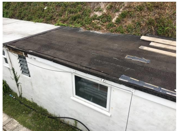
Photograph 6: Showing the exterior of the chalet building with the rendered wall, uPVC window and felted roof visible.
