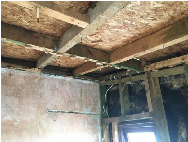
Photograph 1: Showing the interior of the bathroom dormer. The wall of the residential building is visible to the left with the timber frame of the external wall visible to the right. The timber roof structure and chipboard can also be seen above.
