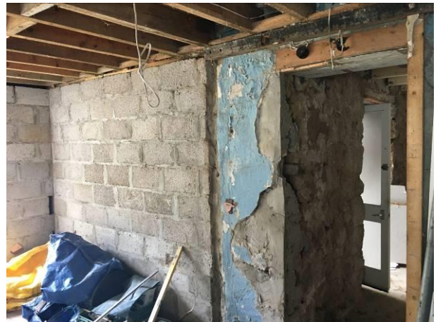
Photograph 10: Showing the interior of the garage with exposed breeze block walls and exposed timber roof structure above.
