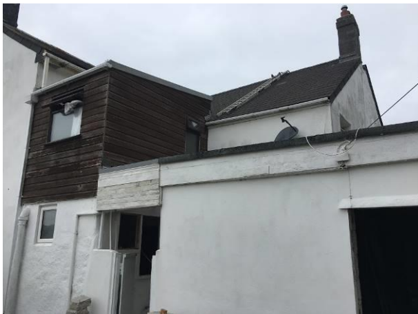
Photograph 9: Showing the garage (bottom right) with the open door visible. The bathroom dormer can be seen to the upper left of the image.
