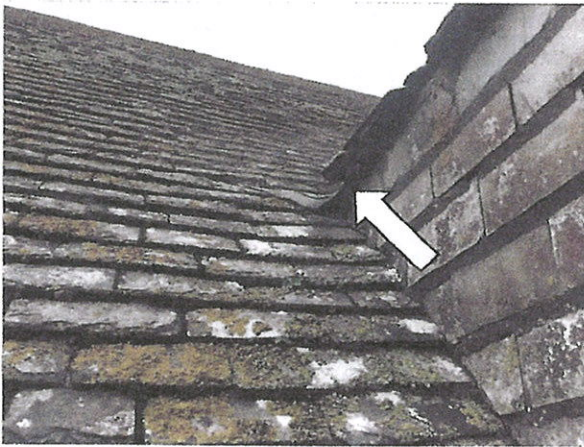
Photograph 3: Showing the location where flashing is lifted at the base of the valley between the dormer and main roof pitches. By contrast, the very tight fit of the remaining scantle tiles and hanging tiles on the dormer can be seen.
