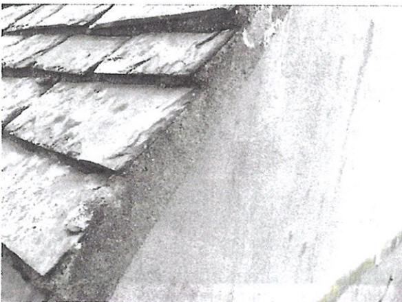
Photograph 5: Showing the tight cement pointing on the roof verge – this is at the gable of No 1 Porthcressa Terrace on the northern aspect.
