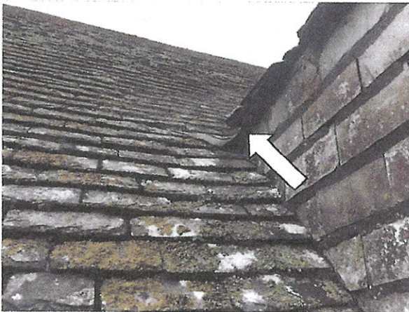
Photograph 3: Showing the location where flashing is lifted at the base of the valley between the dormer and main roof pitches. By contrast, the very tight fit of the remaining scantle tiles and hanging tiles on the dormer can be seen.
