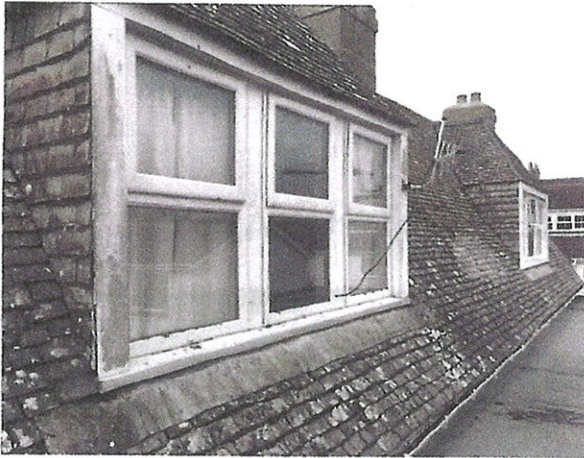
Photograph 1: Showing the pitch of the roof as viewed from the adjacent flat roof.
