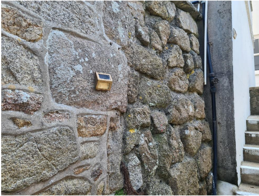
Figure 12: fitting marked for removal.
