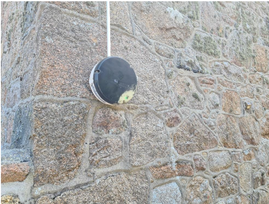
Figure 6: fitting marked for removal.
