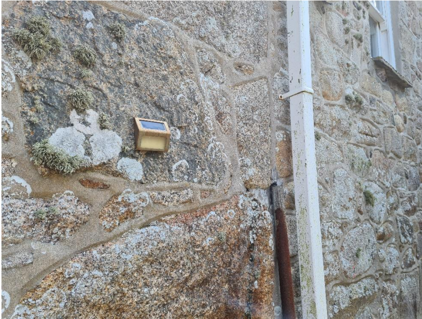
Figure 10: fitting marked for removal.
