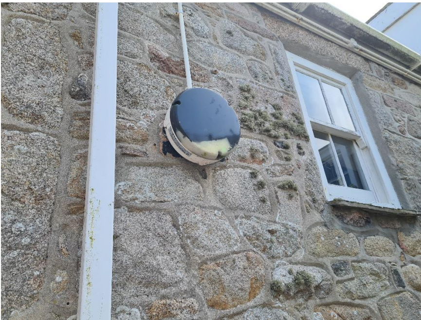
Figure 7: fitting marked for removal.
