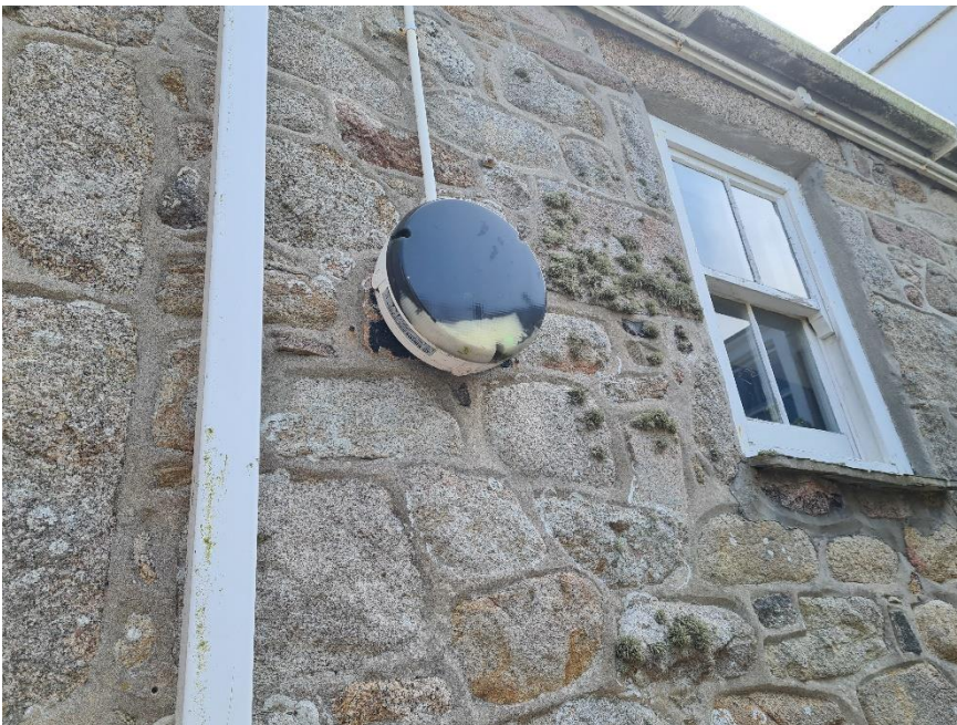
Figure 7: fitting marked for removal.
