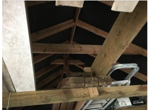
Photograph 10: Showing the interior of the single-storey garage with A-frame timbers and well-fitted underfelting.
