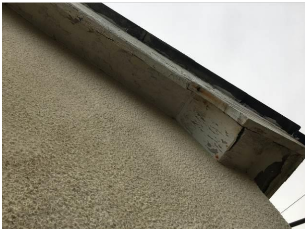
Photograph 3: Showing the good condition of the boxed soffits throughout the majority of the property.
