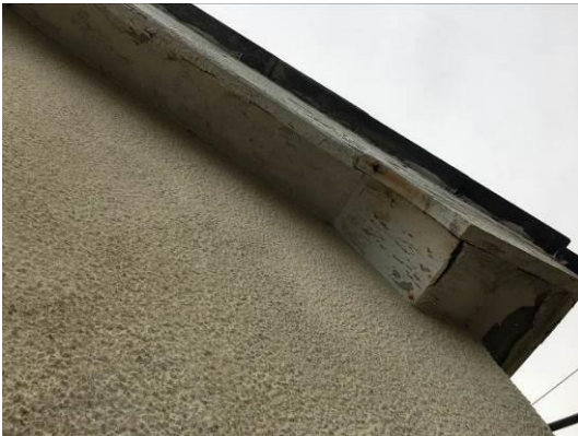
Photograph 7: Showing the good condition of the boxed soffits throughout the majority of the property.
