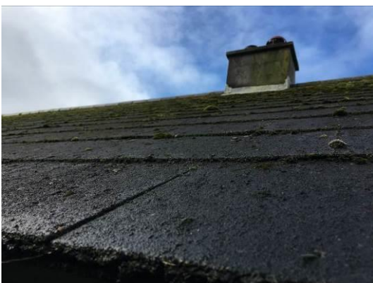
Photograph 9: Showing the tight fit of the roof tiles, with no gaps noted throughout.
