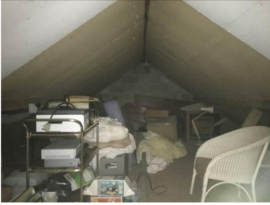
Photograph 11: Showing the interior of one of the boarded out loft components within the property - this example is at the apex but those at the eaves are of equivalent construction.
