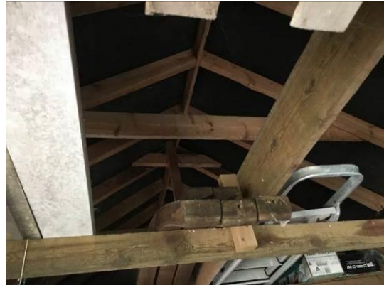
Photograph 14: Showing the interior of the single-storey garage with A-frame timbers and well-fitted underfelting.
