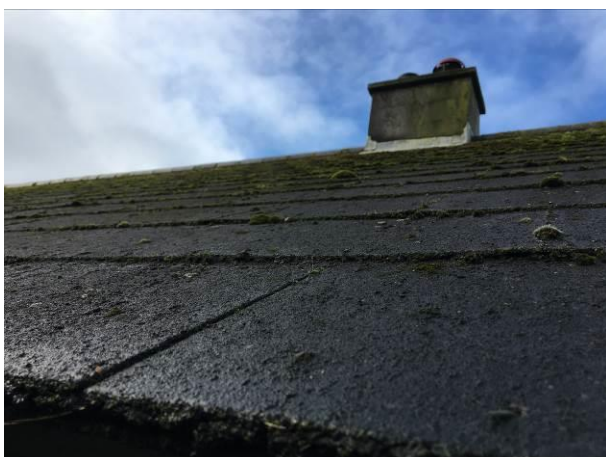
Photograph 5: Showing the tight fit of the roof tiles, with no gaps noted throughout.
