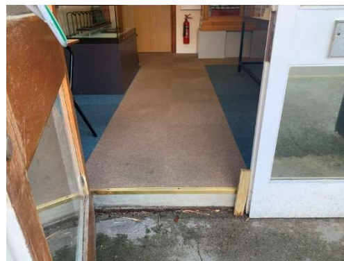
Step at front entrance/exit doors from museum to external footpath.
