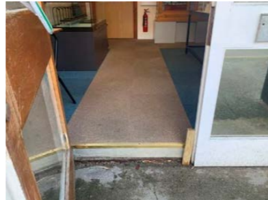
Step at front entrance/exit doors from museum to external footpath.
