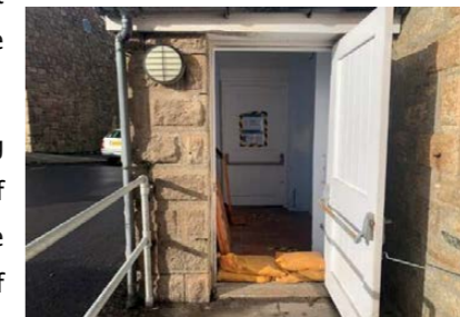
Rear entrance with sandbags across threshold.
