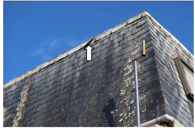
Photograph 8: Showing an example of lifted flashing at the top of the hanging tiles on the 1970's extension.
