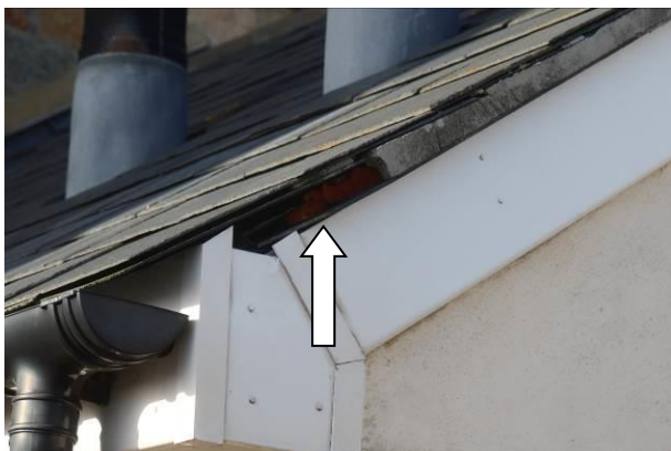
Photograph 5: Showing an example of the gaps allowing potential access beneath slate tiles in the plant room; similar features exist on the rear porch.
