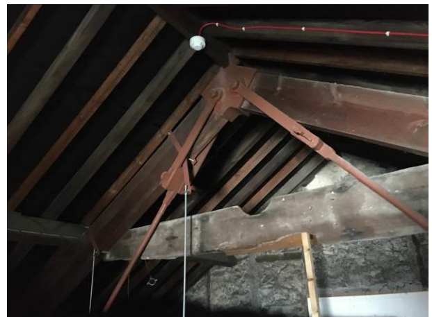
Photograph 12: The attic space within the main hall showing the timber roof structure and underfelting above. Lighting is from the window set into the north wall.
