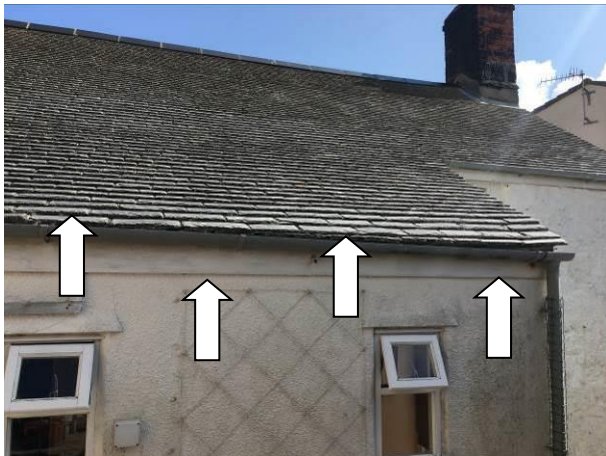
Photograph 17: Showing the northern aspect of the cottage – gaps beneath the tiles at the eaves as well as beneath the fascia boards were noted.
