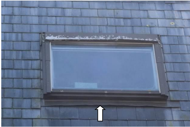
Photograph 1: Showing the lifted flashing around the window on the 1970's extension on the northern aspect.
