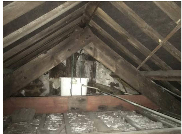
Photograph 18: Showing the loft space in the cottage, viewed from the access hatch.
