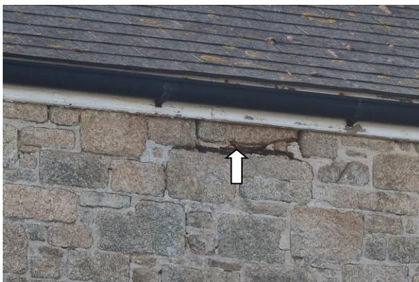
Photograph 3: Showing one of the cracks in the blockwork on the eastern aspect of the hall.
