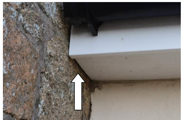
Photograph 6: Showing an example of the gaps allowing potential access beneath soffit box in the plant room; similar features exist on the rear porch.
