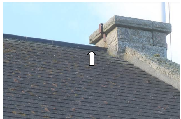
Photograph 4: Showing one of the minor gaps beneath the ridge tiles on the hall.
