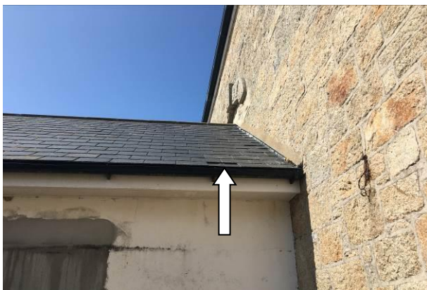
Photograph 9: Gaps under missing tiles on the Plant Room roof.
