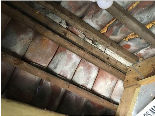
Photograph 13: Showing the internal roof space of the stone shed – this section at the entrance is not under-boarded.
