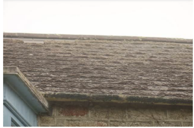
Photograph 2: Showing the tight fit of the roof tiles and abundant moss. The guttering attachment directly to the wall, without soffit or fascia, can also be seen.
