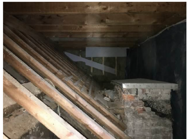
Photograph 4: Showing the redundant northern roof structure sealed within the flat-roof extension on the northern aspect of the building. Accessed and visible from the loft space of the property.
