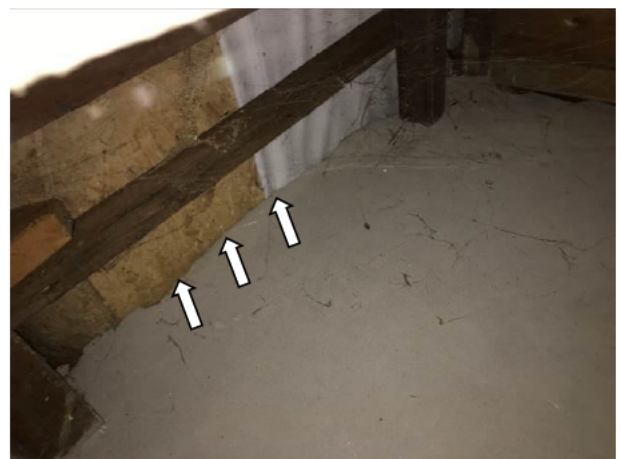
Photograph 6: Showing the concrete wall between Camelia and Magnolia Cottages with minor gaps at the top which a bat could potentially use to access between the loft spaces.
