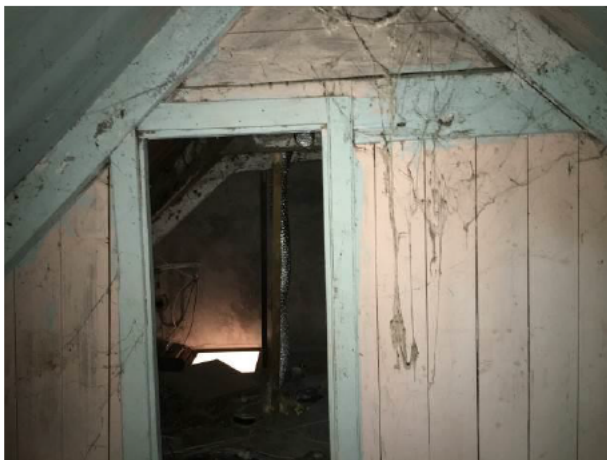
Photograph 3: Showing the timbers which underboard the loft space and also create an internal partition.
