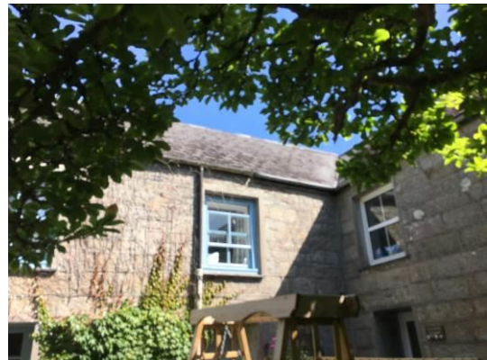
Photo 04 – Showing Magnolia Cottage from the exterior. The southern and western pitches of the roof can be seen.
