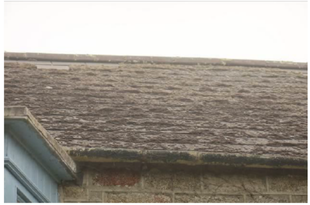
Photograph 2: Showing the tight fit of the roof tiles and abundant moss. The guttering attachment directly to the wall, without soffit or fascia, can also be seen.
