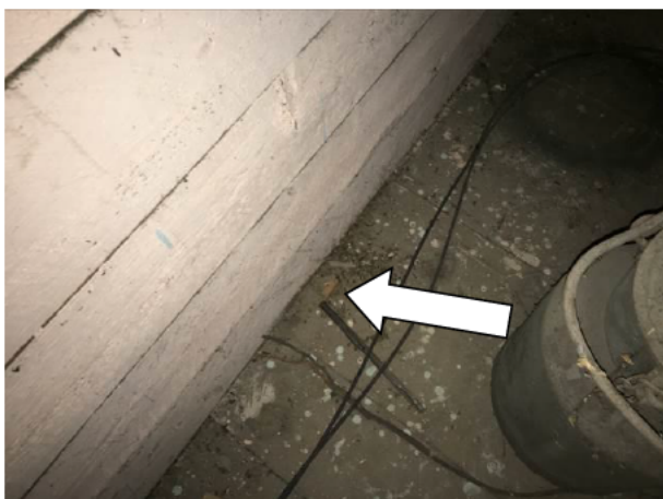
Photograph 5: Showing the accumulation of droppings – primarily rat and mouse with individual droppings characteristic of brown long-eared bat – at the western end of the loft space. The confirmed bat dropping was identified suspended in a cobweb immediately above this.
