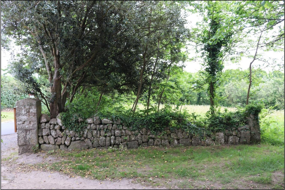
FIGURE 12: THE NORTH-WEST BOUNDARY WALL, BUILT AGAINST A SQUARE, GRANITE GATE PIER, VIEWED FROM THE WEST.
