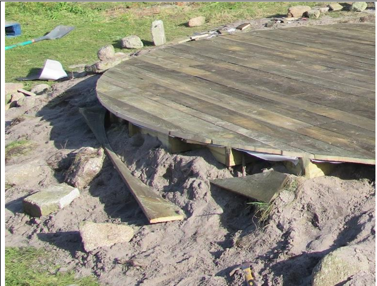
Photo 2 – showing the base of the yurt during construction. The elevation above the surrounding land can be seen.
