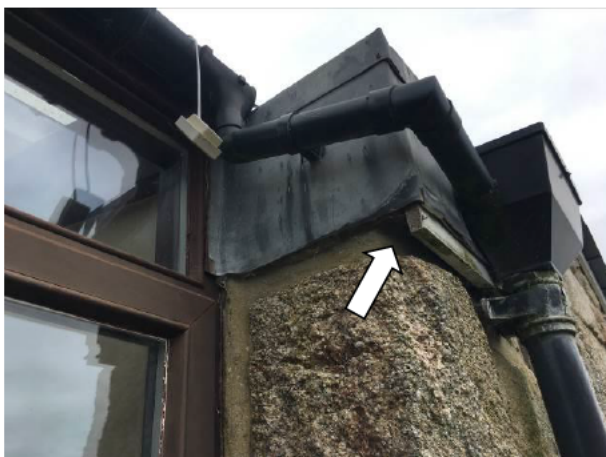
Photograph 5: Showing the gaps in the adjacent fascia and flashing on the single-storey aspect of the building.
