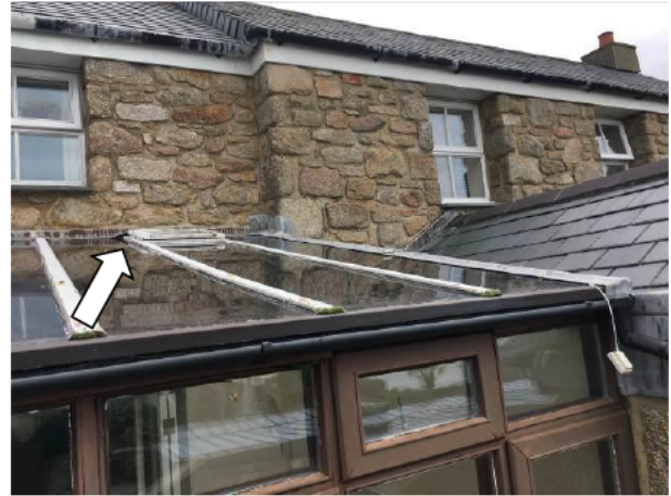
Photograph 2: Showing the roof of the conservatory – the flashing at the junction with the house can be seen with very minor gaps indicated.
