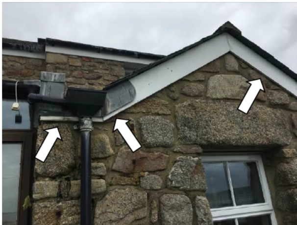
Photograph 3: Showing the proximity between the fascias on the gable of the single-storey structure (indicated) and the conservatory to the left.
