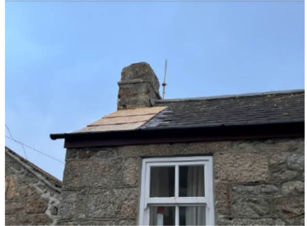
Photograph 2: Showing roof with the temporary repair to the damaged section below the northernmost chimney
