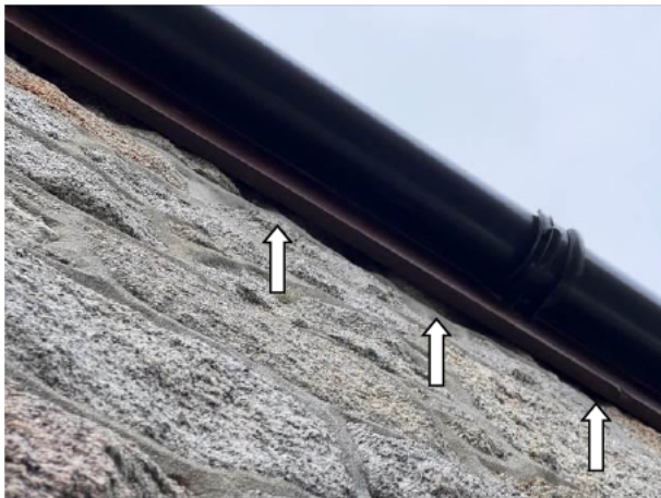
Photograph 3: Showing the fascia board with intermittent gaps behind.
