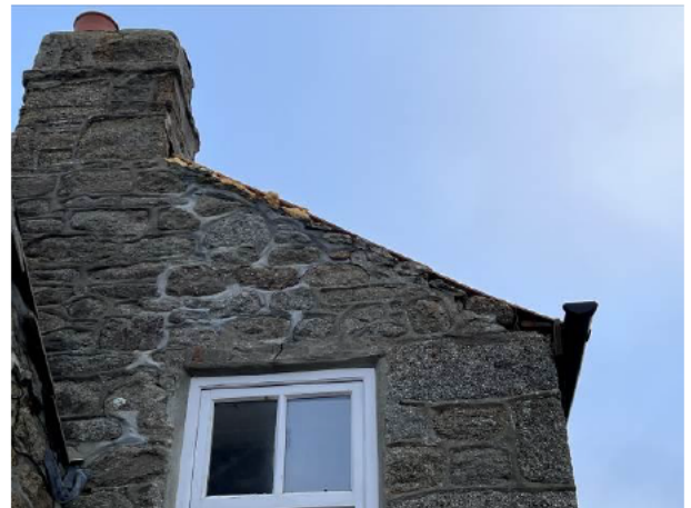
Photograph 4: Showing the northern gable with the expanding foam associated with the temporary roof repair visible above the verge.
