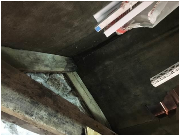
Photograph 5: Showing the interior of the stable block – the terminal roof timbers can be seen abutting the granite gable wall. The underfelting is generally intact.
