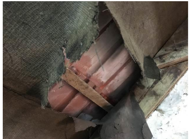
Photograph 6: Showing a gap in the underfelting where the tiles can be seen, attached directly to battens.
