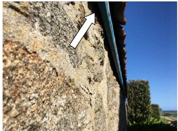
Photograph 4: Showing an example of gaps beneath fascia boards on the building – these were fully inspected with a torch or video endoscope.
