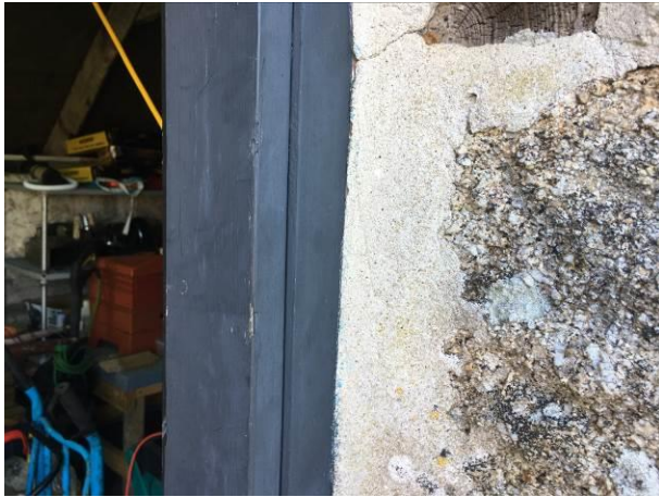
Photograph 7: Showing an example of the pointing where the door frame meets the walls – no gaps were identified.
