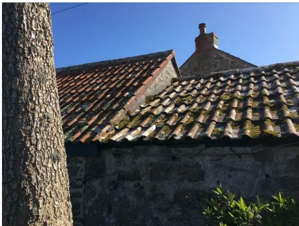
Photograph 3: Showing the location where the stable block (left) adjoins the offsite outbuilding (right)
