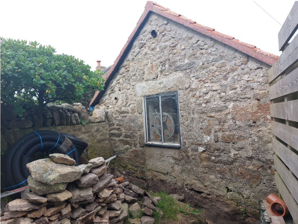
Photo of the gable end of the Stables from the garden of Signal Rock.
