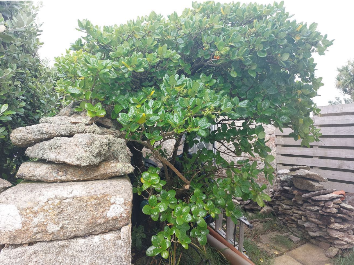
Photo of the boundary wall between the Stables and the paved lane.
