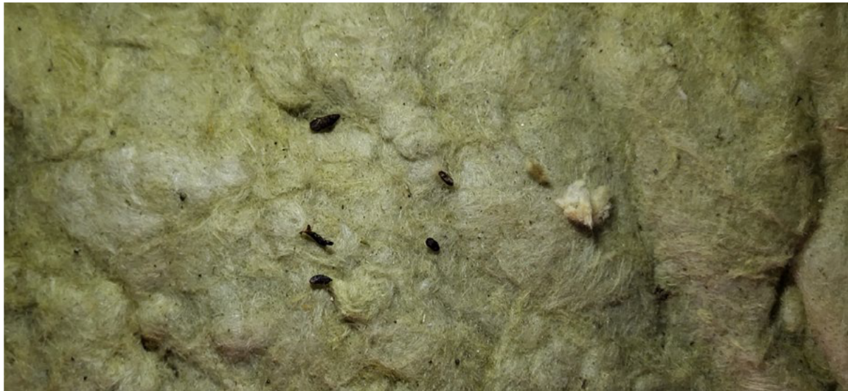
Figure 9: Droppings on roofing insulation of roof void 3
