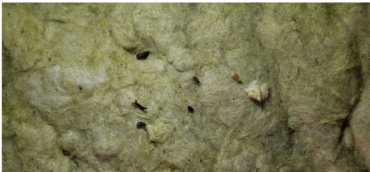
Figure 12: Droppings on the roofing felt close to the hatch entrance of roof void 3
