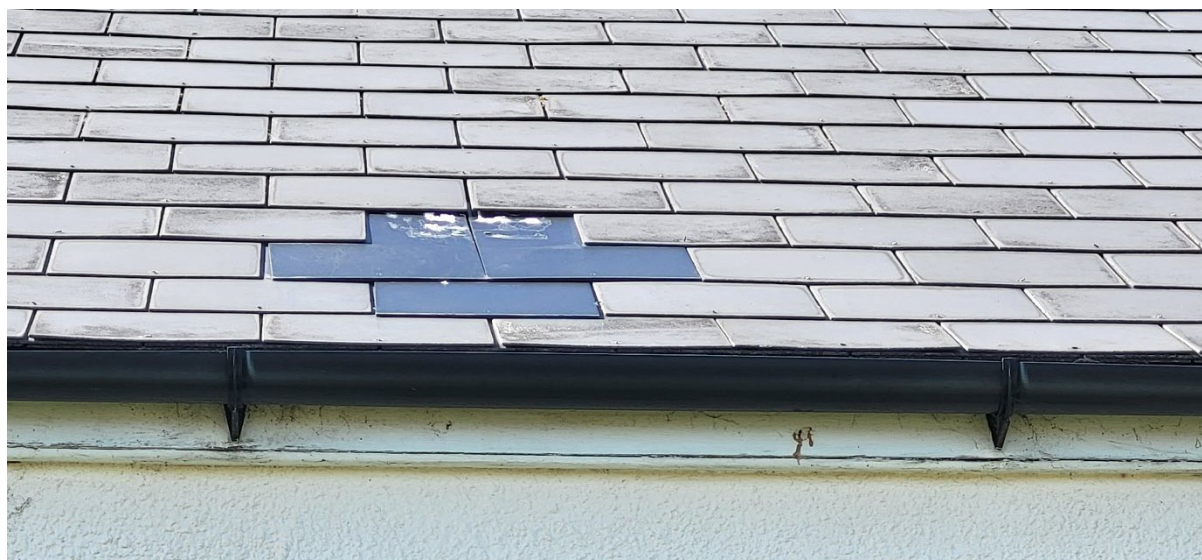
Figure 9: Replacement roof slates on the east elevation that may provide an access point for bats
