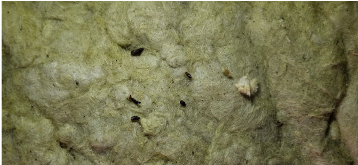
Figure 9: Droppings on roofing insulation of roof void 3
