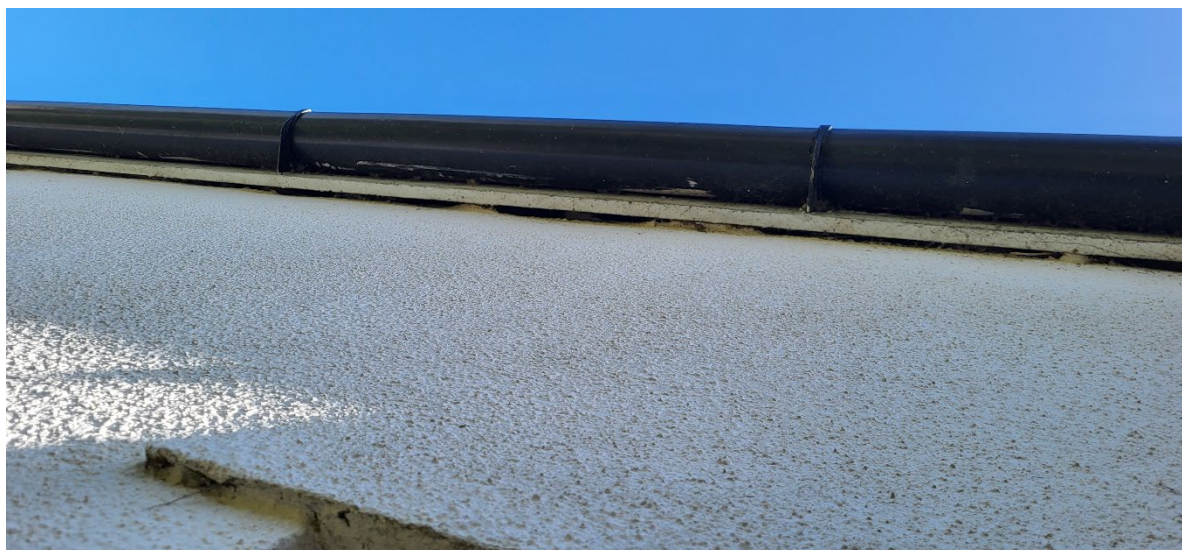
Figure 8: Gaps behind the fascia boards on the west elevation
