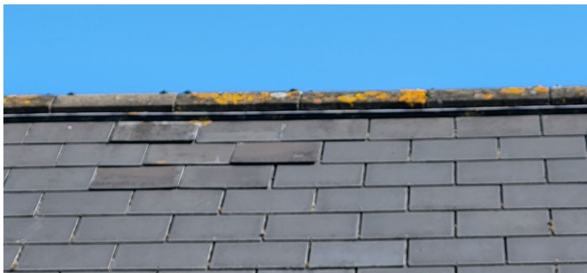
Figure 7: Raised roof slates on the west elevation of Bottom Annexe
