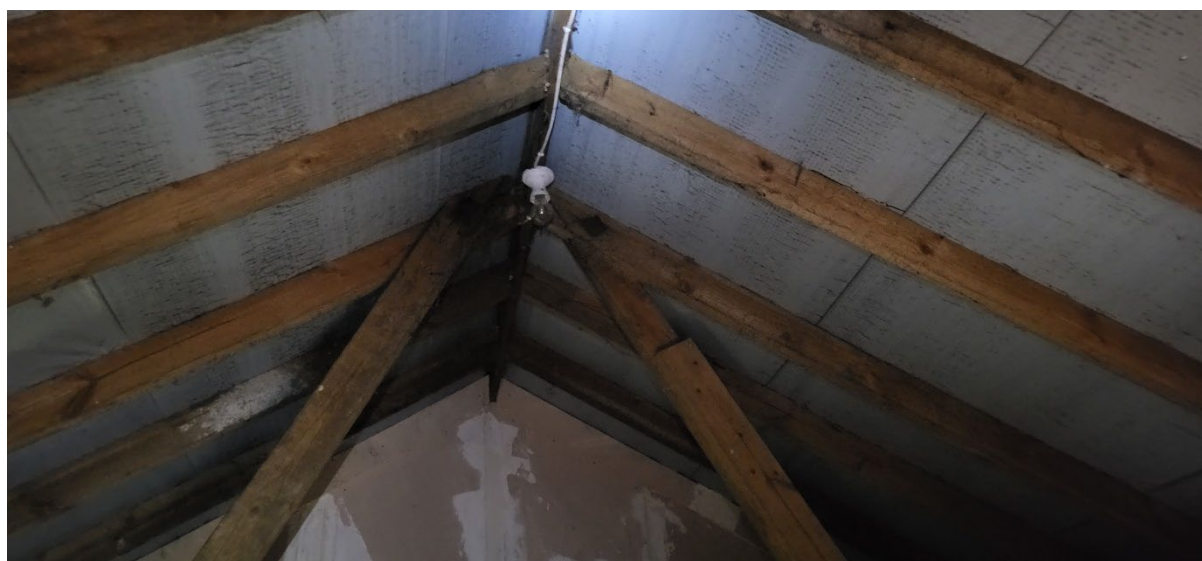
Figure 10: Roof structure of roof voids 1 and 2. Impermeable plastic liner and timber frame
