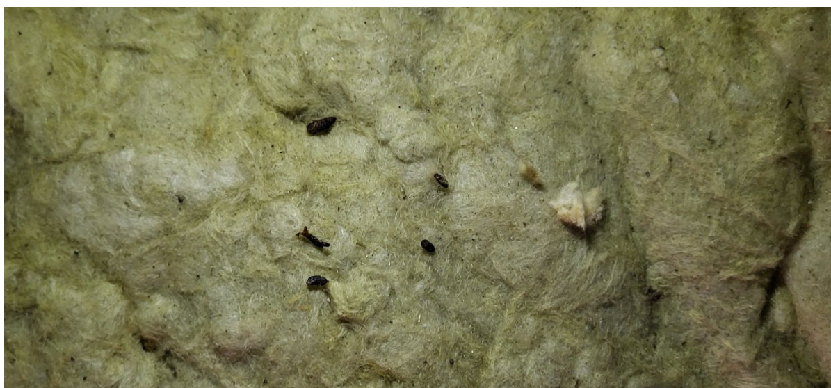
Figure 12: Droppings on the roofing felt close to the hatch entrance of roof void 3
