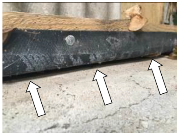
Photograph 4: Showing the minor gap occasionally present between the top of the wall and the timber wall plate.
