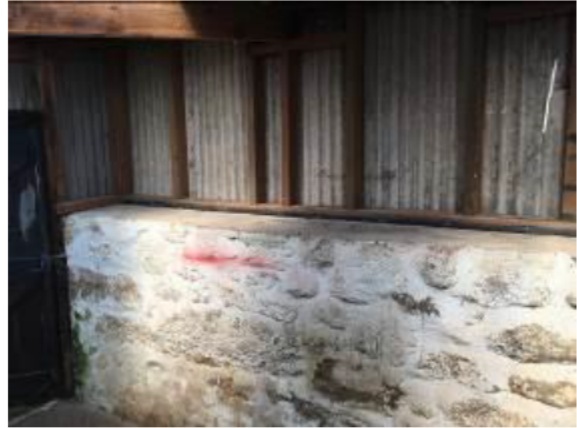
Photograph 2: Showing the typical internal structure, with the stone-block wall supporting a timber frame with corrugated sheeting attached.
